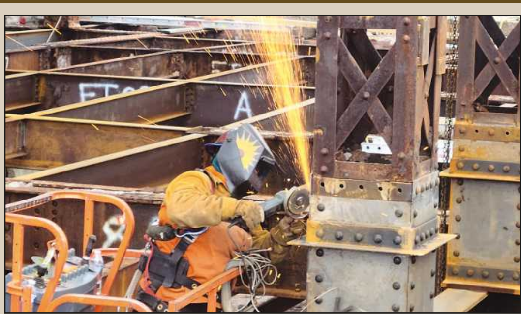
MAKING SPARKS FLY earlier this year while re-constructing the base of one of 14 lattice-steel columns at the Michigan Central Train Station project in Detroit is Tiffany Younk of Iron Workers Local 25. The rotted steel on the lower column was replaced with new, while the original 1913 riveted lattice steel above has been mostly retained. The iron worker crew on the project is employed by Midwest Steel.
